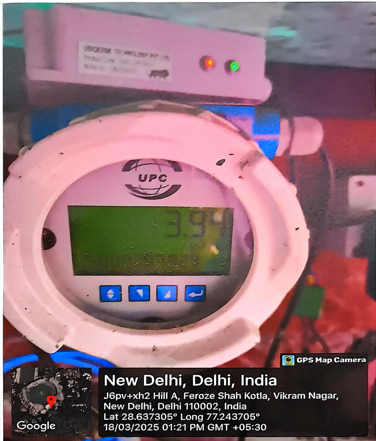
Water Flow meter (flow rate 3.94m 3 /hr)
