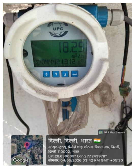
Water Flow meter at Tubewell No.2
